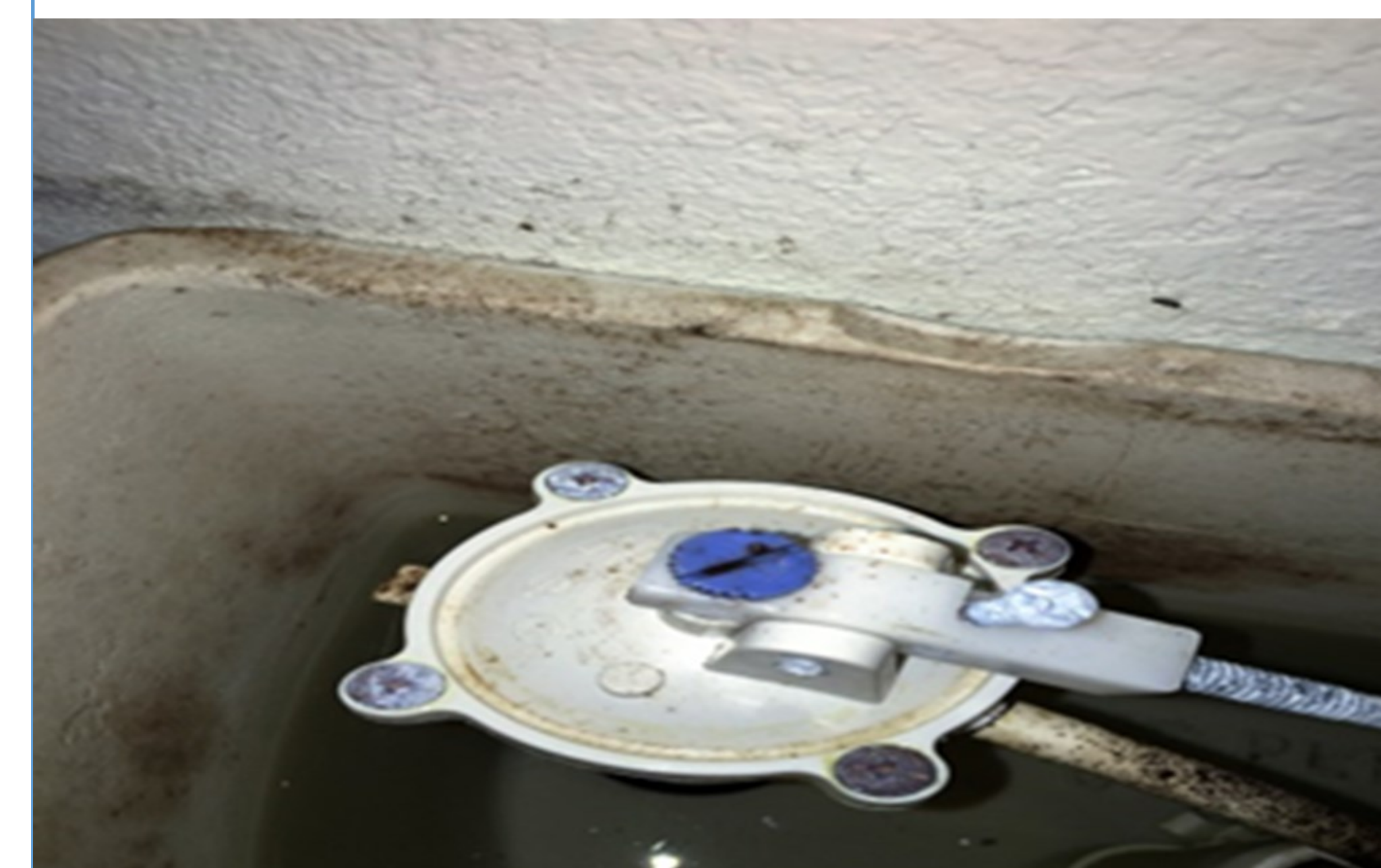
Fig. 1. The accumulation of mold in a toilet
