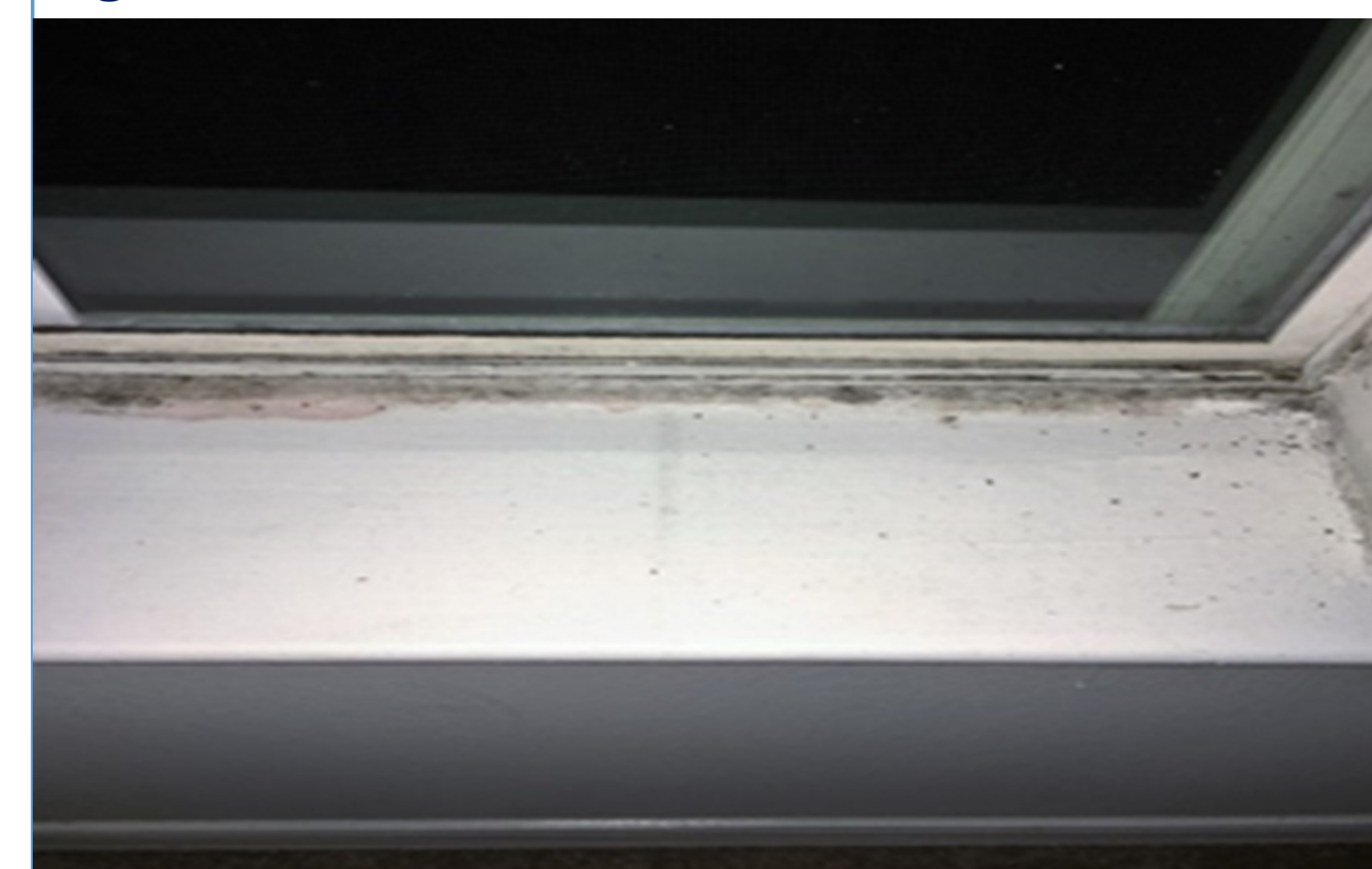
Fig. 2. Mold on a window sill
